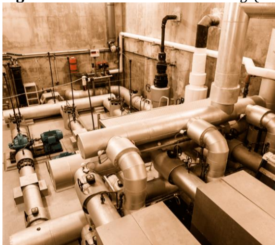
Figura 7: Sea Water Air Conditioning (SWAC) do hotel The Brando
